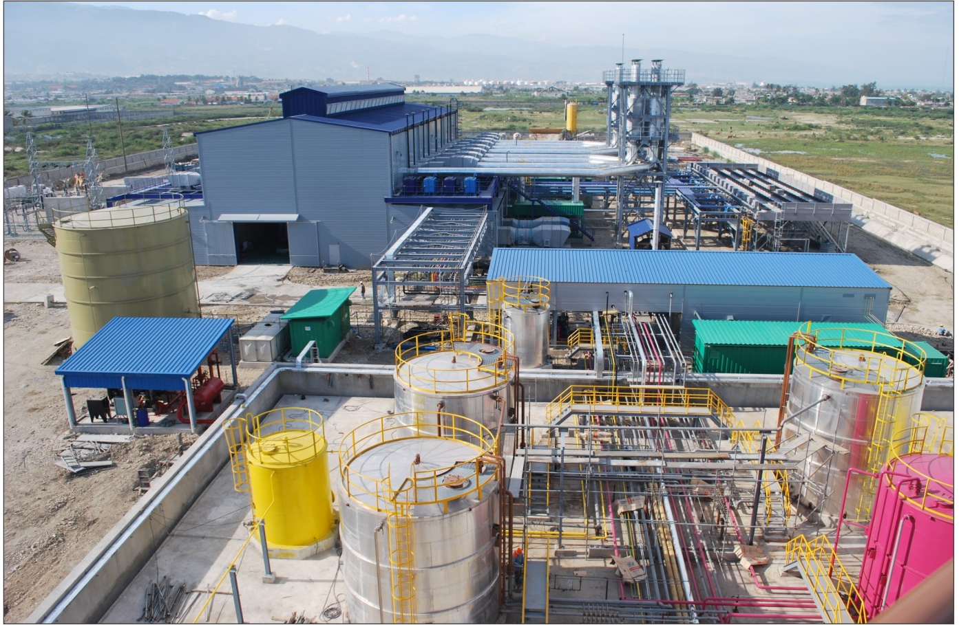
Heavy Fuel Oil Power Station—Haiti
